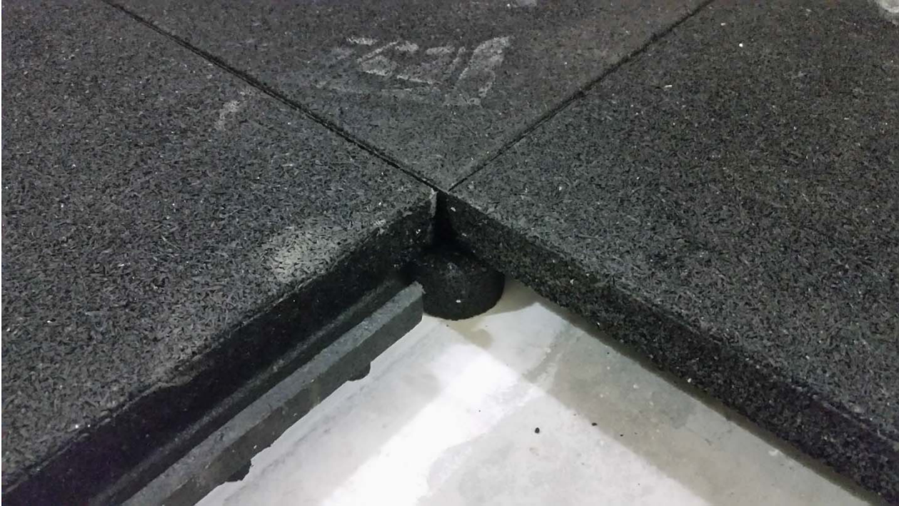
Figure 3 – Typical support pedestal installation
